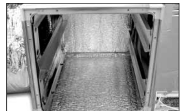
7. Remove filters and secure via panel from inside to the air handler
